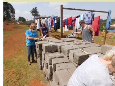
Some Of Our 2017 Team Wire Brushing All The Solid Block In Preparation For Laying The Retaining Wall Behind The Kitchen.
